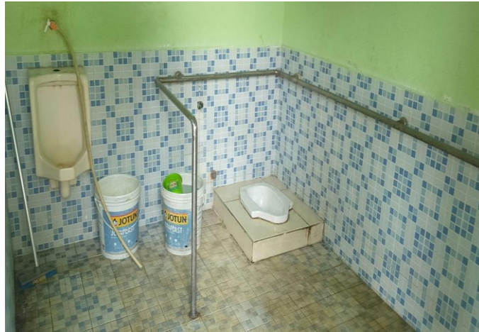
Figure 5-21 The ongoing construction of an inclusive toilet in the Krendang community park initiated by the project 16
